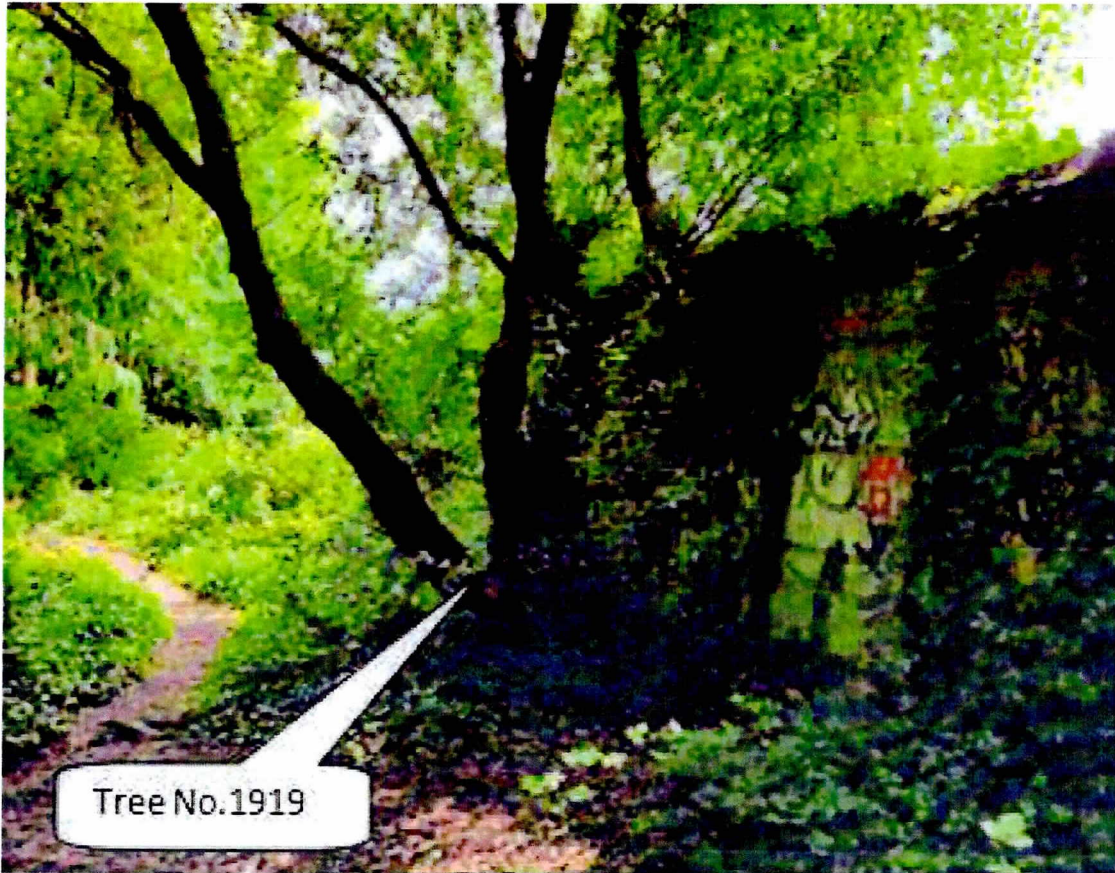
Figure 6 Photograph No. 3: shows Tree No. 1919 growing tight to the boundary wall, but shown on the tree survey drawing in a different location and marked for retention.
